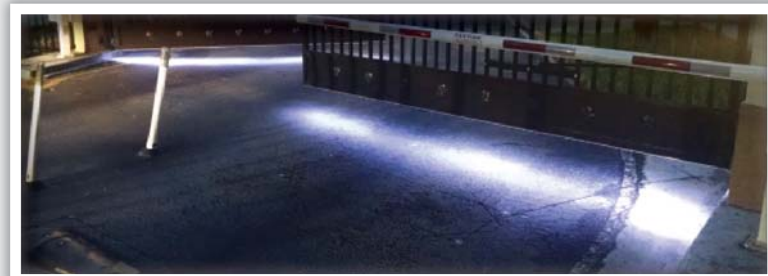
Slide gate lighting is mounted to the fixed entry posts on left and right of the entry.
